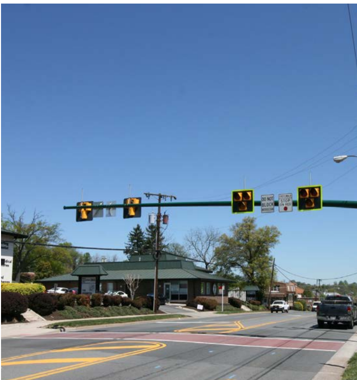
Pedestrian Signals: HAWK signal at the mid-block of the 300 block of Maple Avenue West
