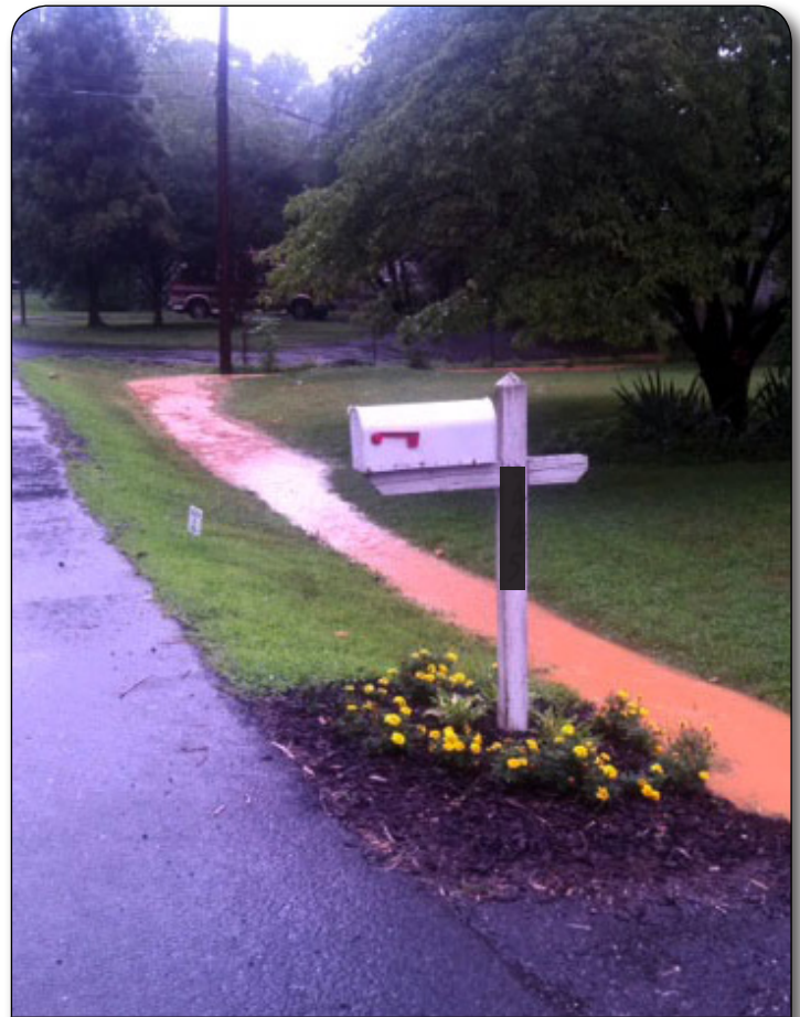
Run-off has become an issue with the increase of new homes being constructed in the Town
