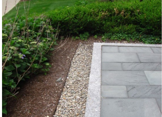
French Drain collecting Runoff from a Patio (Photo courtesy of University of Rhode Island)
