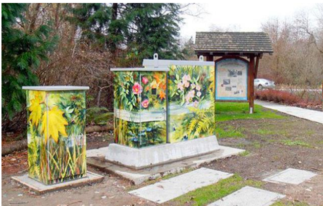
Fig 8.3.0: Example of utility box wrap - Bellevue, WA
