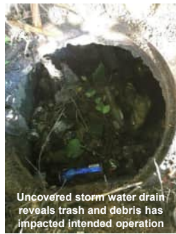
Illegal Dumping of Cooking Oil/Grease, Trash and Debris
